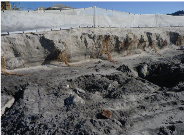
Photo 6 The same area after storm damage. Photo credit: F. Gesing, July 2011
