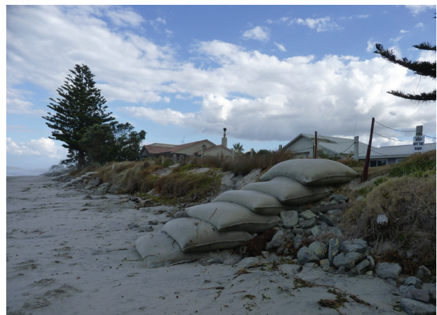
Photo 7 The area four years after the dune enhancement, with geotextile bags as temporary access structures. Photo credit: F. Gesing, February 2015
